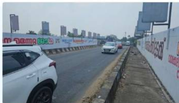
Drain outlets are clogged in the section above the railway crossing
