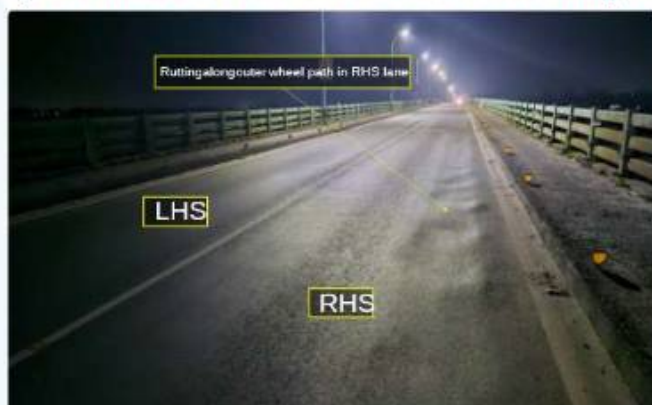
Shoving along the outer wheel path in RHS lane in Alexander Parambithara Bridge
